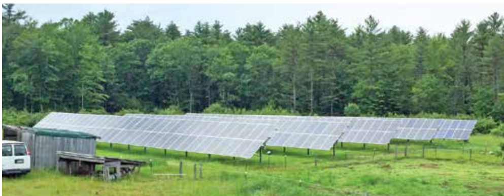
Bob’s Clam Hut Community Solar Farm (Hollis, ME)
